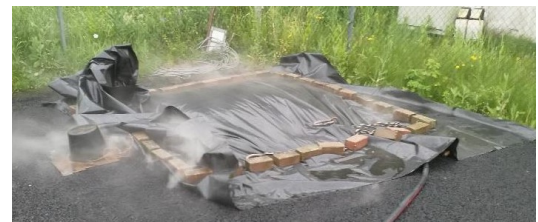
Steam Heating set up
